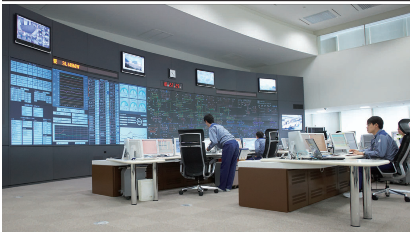
The Central Load Dispatch Center monitors fluctuations in power demand and issues instructions to power plants in each region on required output levels.
