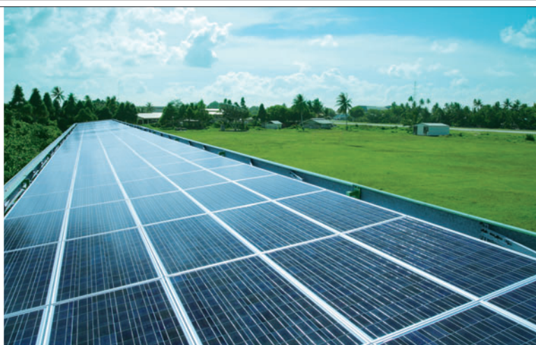
Tuvalu: Solar Power Project
