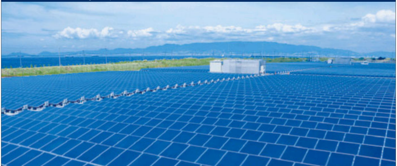
Sakai Solar Power Station, a mega solar power plant
