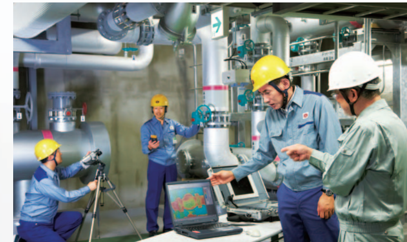
Energy efficiency diagnosis
