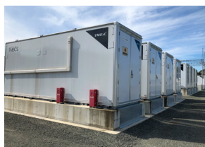
Example of grid scale batteries we developed (Kinokawa Energy Storage Plant)
