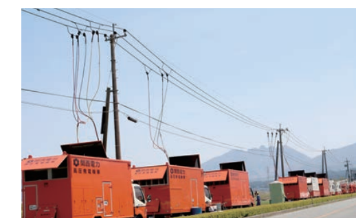
Emergency power transmission with high voltage power generators (Image is for illustrative purposes.) (April 2016)
