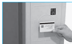
Monitoring electric locking/unlocking of doors and entrance and exit history
