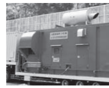
Air-cooled emergency generator
