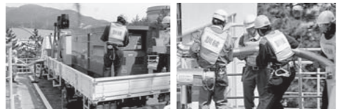
Installation of a medium-pressure pump to supply water to the steam generator
