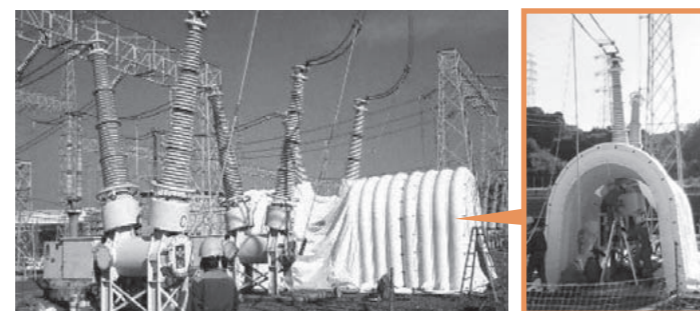
Gas circuit breaker
