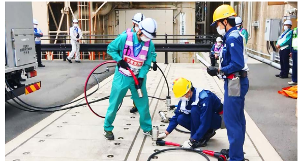
Training on transportation and connection of Chugoku Electric Power's high-voltage power supply vehicle
