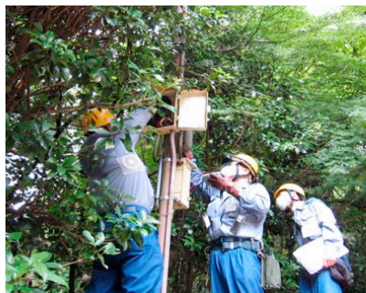
Electrical equipment inspection at Shoshazan Engyoji Temple, Hyogo
