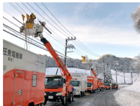
Emergency power transmission with generator vehicles (December 2020)
