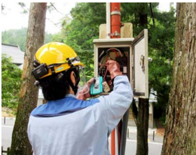
Electrical equipment inspection at Mt. Koya, Wakayama
