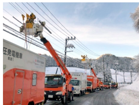
Emergency power transmission with generator vehicles (December 2020)
