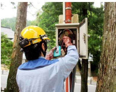
Electrical equipment inspection at Mt. Koya, Wakayama
