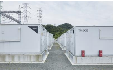
Kinokawa BESS Plant (COD in 2024)
