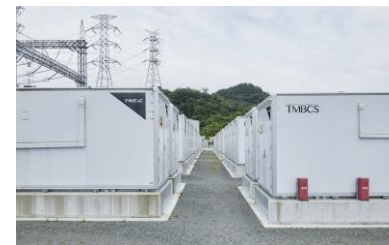
Kinokawa BESS Plant (COD in 2024)
