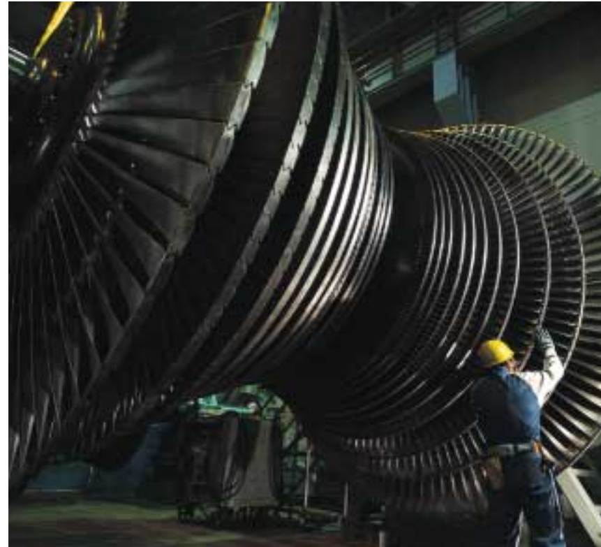
Periodic inspection of nuclear power plant turbines. By shortening inspection intervals, the company is working to trim costs and boost utilization ratios.
