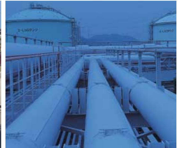
LNG base at Himeji No.2 Power Plant. It serves as the base for companywide gas operations.
