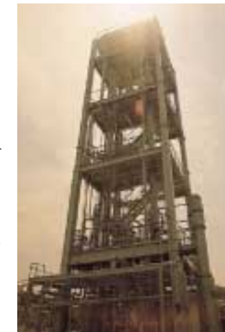
Flue-gas decarbonization pilot plant set up within Nanko Power Plant. Research is under way into recovery of CO 2 present in power-plant flue-gas emissions.
