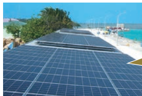
Solar power generation facility that we transferred to Dhiffushi Island in the Maldives
